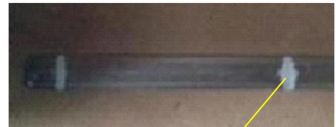
Fuel Oil Level Mark
