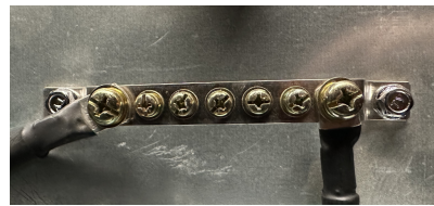
Generator Grounding Bar Lug.
